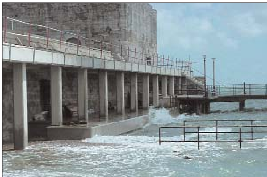
Pictures show the renaissance of Portsmouth Harbour, part of the Millennium Landmark Project. The contract involves a partnering agreement, evolved from Best Value.
